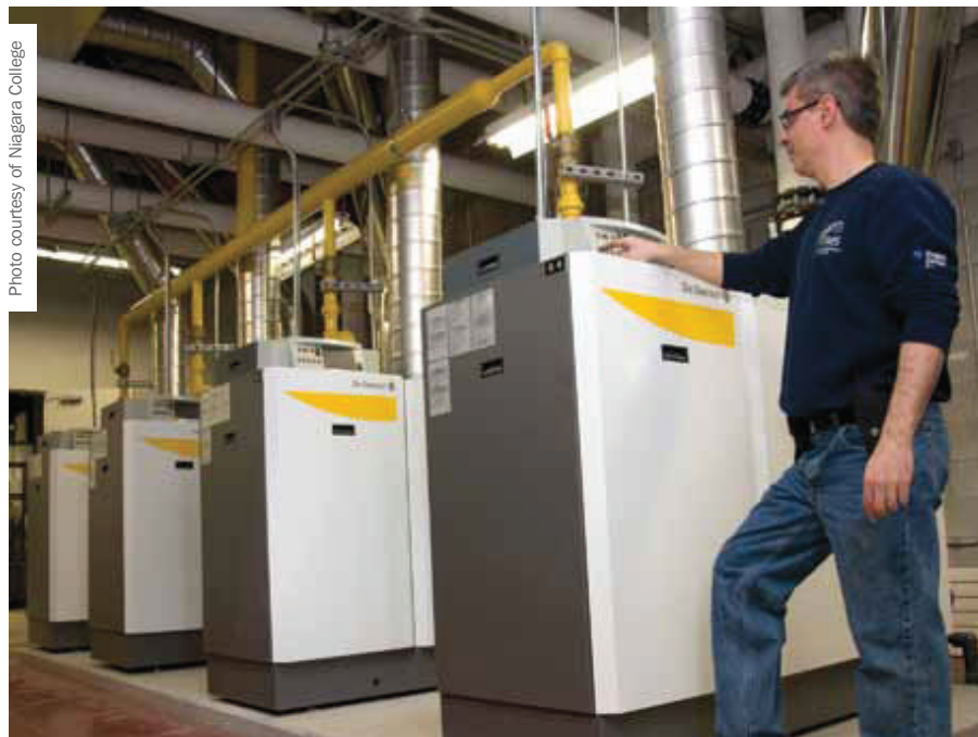
Pat Vilella of Niagara College adjusts controls of recently upgraded boilers at the Welland campus.
